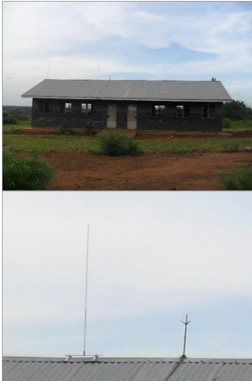
Fig. 4. Upper photo: Classroom building at Runyanya School. Lower photo: Closeup showing IEC compliant rod and old multipronged rod commonly found on many Uganda schools that ACLENet staff have visited and measured.
