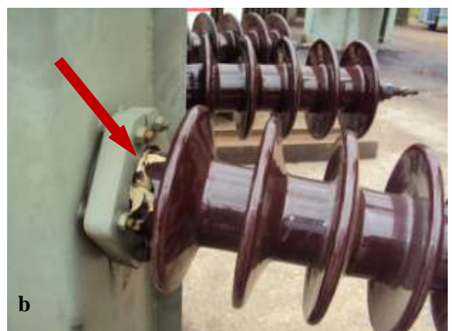
Figure 3 a. Damaged transformers in the ZESCO yard in Mkushi b. Damaged part of the transformer
