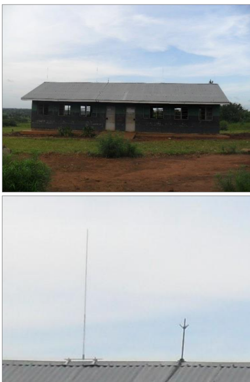
Fig. 3. Upper photo: Classroom building at Runyanya School. Lower photo: Closeup showing IEC compliant rod and old multipronged rod commonly found on many Uganda schools that ACLENet staff have visited and measured.
