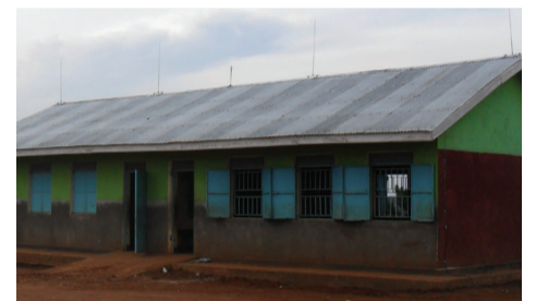
Figure 2. Runyanya school building where 18 students were killed and 38 injured by lightning in 2011. Note the multiple Franklin rods on the roofline with the old multi-prong shorter rod in the center.
