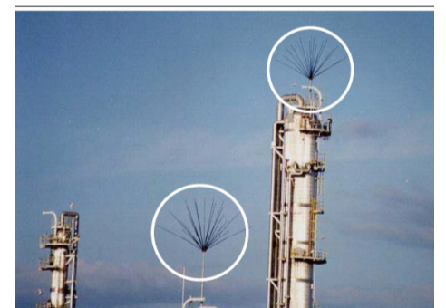
Figure 4. SLE (Semiconductor Lightning Eliminator) air terminals (circled) installed on petrochemical processing plants. Their claimed ability to reduce the 'captured' lightning current by 99% has been disproved by scientists
