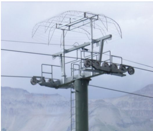
Figure 7. Multiple varieties of 'enhanced' lightning arrestors.
