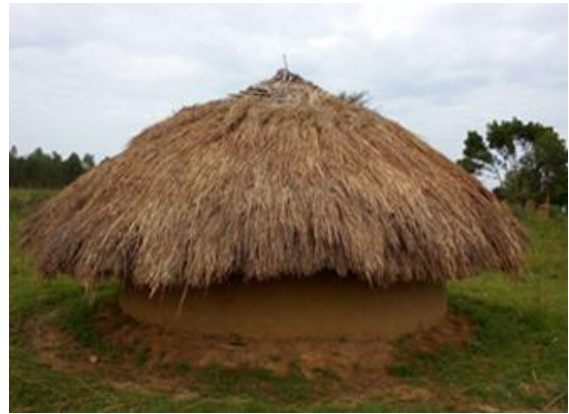
Fig. 2. Most of the children who were injured were sitting a small veranda around this unfinished hut, taking shelter from a drizzle. The top center point of the roof was not yet thatched, remaining open so that rain and sunlight could penetrate to the inside.
