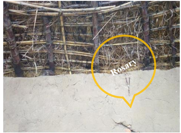
Fig. 4. Photo of the wall where thatch roof meets the mud wall. The inside was scorched by fire apparently started by lightning. A rosary was hung to chase away evil spirits
