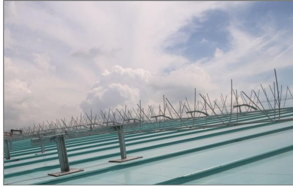
Fig. 17.6 ‘Lightning Eliminators’ – Not accepted by any lightning standard (courtesy HCFP Pte. Ltd.)
