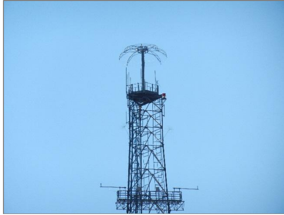
Fig. 17.5 Two ESE air terminal designs (photos courtesy National Lightning Safety Institute)
